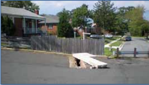
Cover pushed off storm drain
