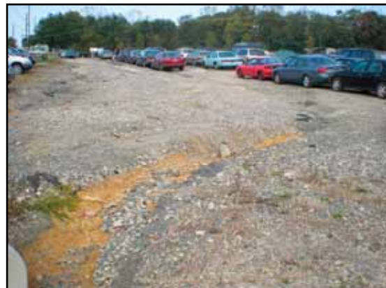
Parking lot erosion at the auto auction along Beech Road
